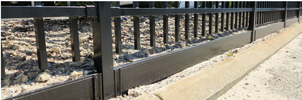
Garrison Security Fencing - with Retaining Plinth
